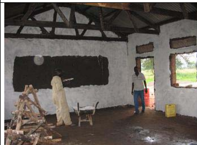
Inside slab and wall plastering is done on one room. Windows will be fixed next week.
