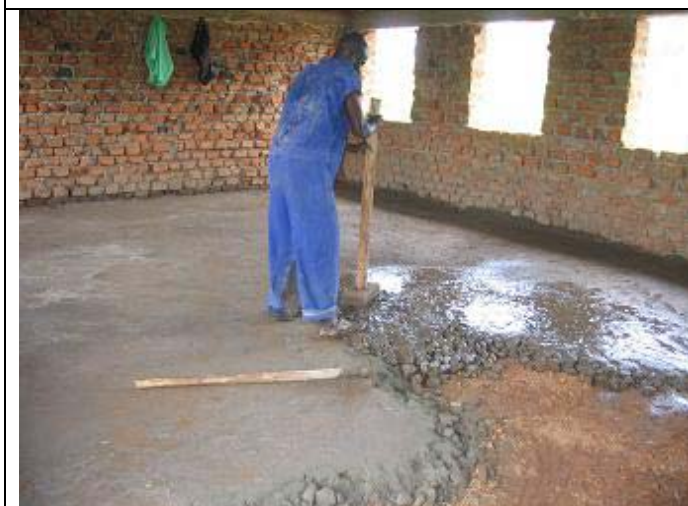
One of the builders is pressing or laying concrete (slab) in one of the classrooms.
